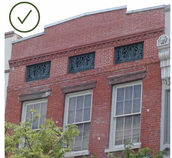
Because this buildings flat roof is screened by a parapet wall, it may be of any material.
