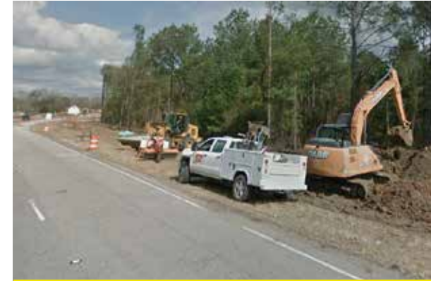
Construction of shared-use path on Henry E. Brown, Jr. Boulevard between Liberty Hall Road and Red Bank Road.
